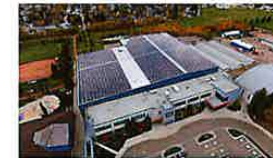
Camrose Rec Centre Solar Array
