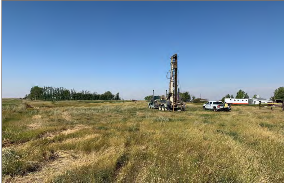
Photo 5: View looking westerly at the central portion of the site. The drill truck was being used for a geotechnical evaluation for the site.
